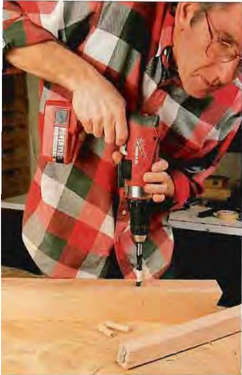
Transfer the dowel hole locations using dowel centers. A slight tap on the top of the legs drives the center point of the dowel center into the beam. Then drill the holes.
