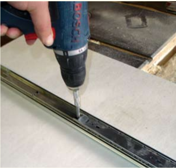
STEP THREE By first installing the upper drawer slide on the bottom of the top shelf, I was able to locate the shelf at exactly the correct height in the cabinet.
