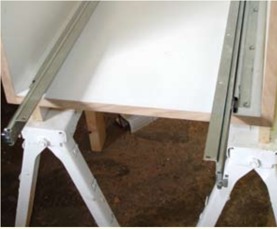
STEP ONE First, I installed the lower guides in the bottom of the cabinet.
