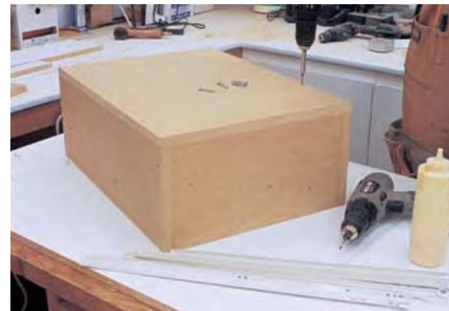
STEP 13 The lower middle drawer box is 8\frac{1}{2} " high by 16" wide by 22" deep. Build the box using \frac{3}{4} " MDF with parts T, U and V following the same steps as the outside lower drawer boxes. Mount this box using 22" drawer glides.
