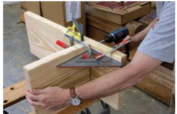
Square to start. Square subassemblies will make the overall structure easier to put together.
