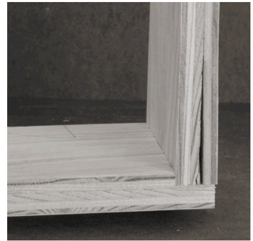
Fasteners driven in the edges of plywood can cause an inferior core to split, often delaminating adjacent layers.
